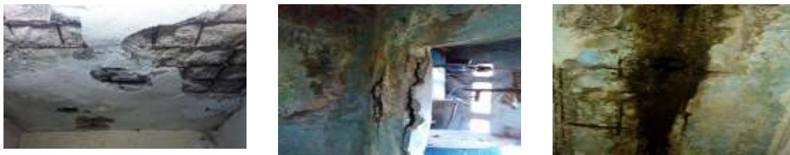
Fig. 2. Elements showing the corrosion of steel.
